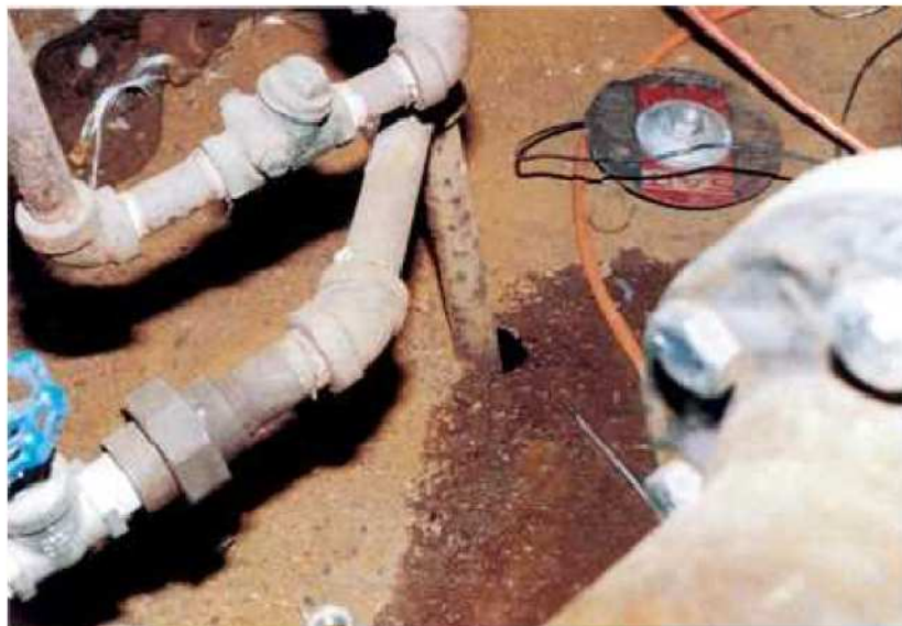
Figure 2: The external piping restraint caused surface cracking inside the vessel.
