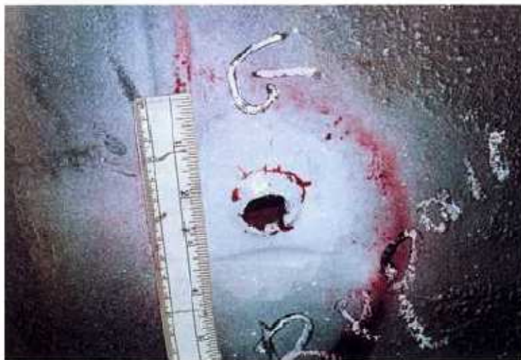
Figures 3 and 4: Lack of penetration is just one cause of this type of cracking.
